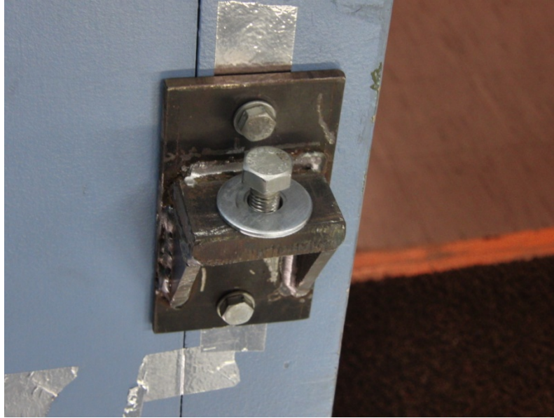
Figure A-1 Bracket placed on the tunnel wall next to the access door.
